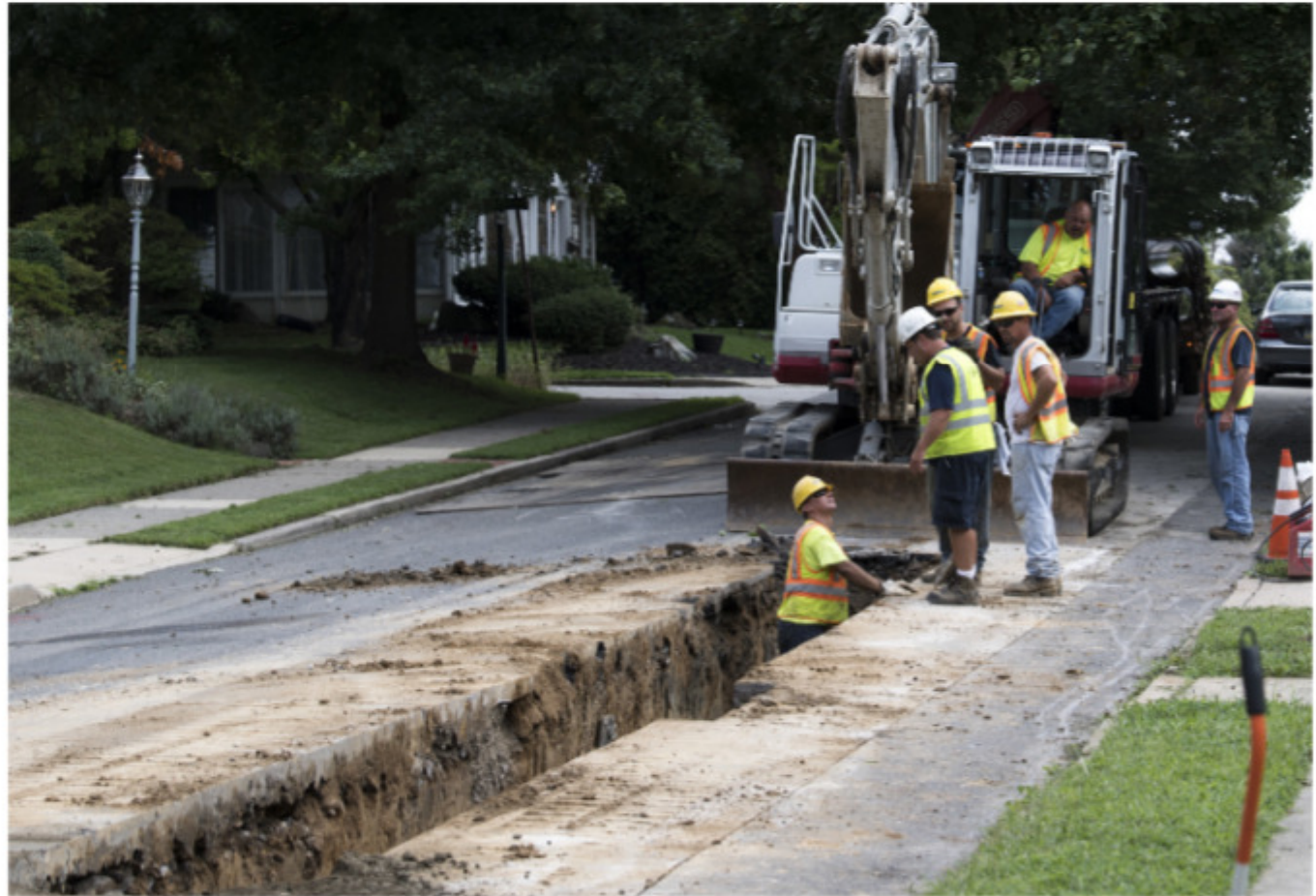
Aqua Pennsylvania contractors rebuild a water main on Hillcrest Road in Upper Darby. Pennsylvania laws on selling public water and sewer systems to private companies need to be revamped, Bill Ferguson writes. Jose F. Moreno / Inquirer File
